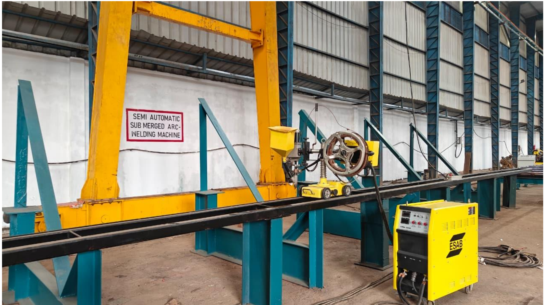
SEMI- AUTOMATIC SAW WELDING MACHINE
